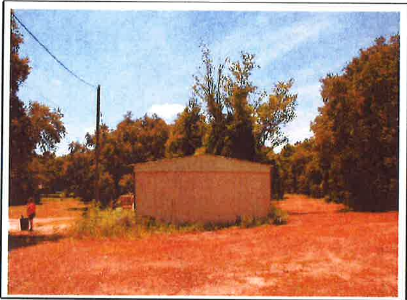
(5) Westerly (side) view of the subject residence. Photograph taken by Thomas A. Riddle, MAI on July 30, 2014
