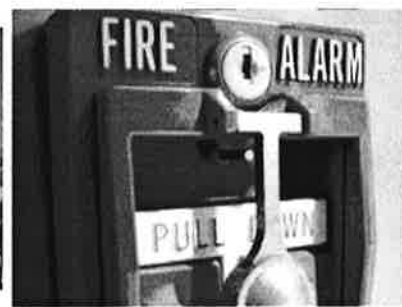
Fire Alarm & Safety
