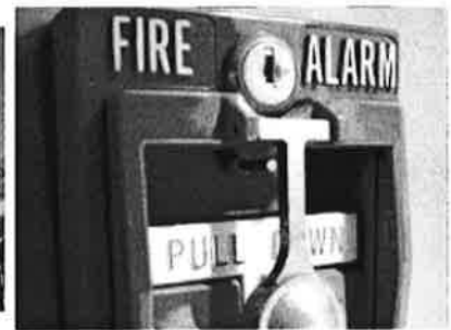
Fire Alarm & Safety
