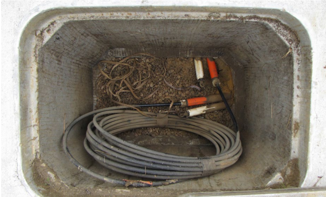
Figure 1.3: Fiber pull box
