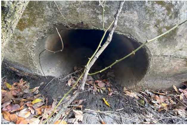
Downstream of 19" x 45" ERCP crossing Dallas Blvd just north of the on-ramp. (facing east)
