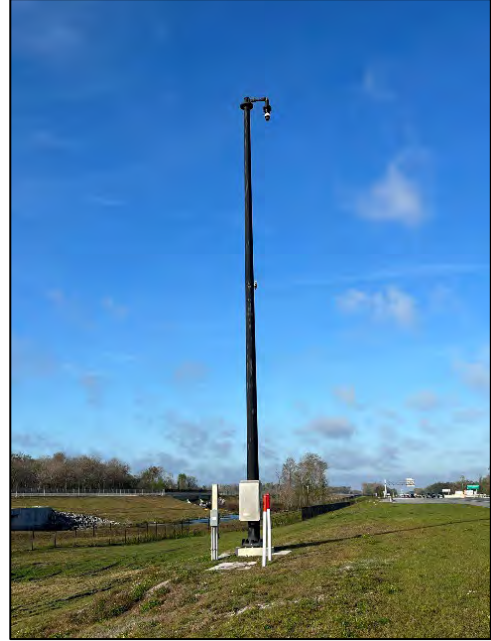
Figure 14 - Device 2 (CCTV MM 23.2)
