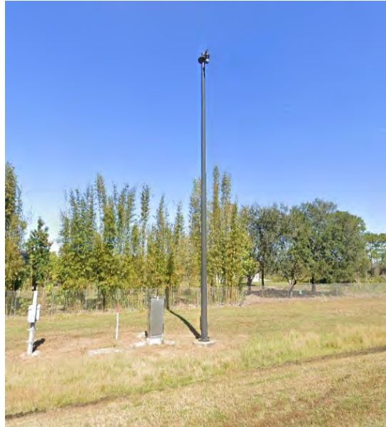
Figure 21 - Device 11 (CCTV, MM 24.5)
