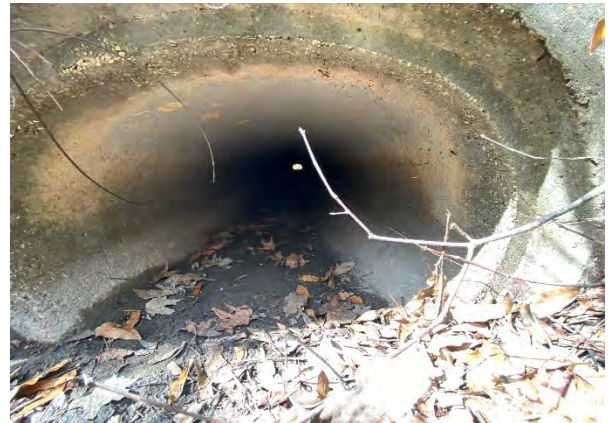
Inside pipe on upstream side of 19" x 45" ERCP crossing Dallas Blvd just north of the on-ramp. Good condition. 2" of silt. (facing west)
