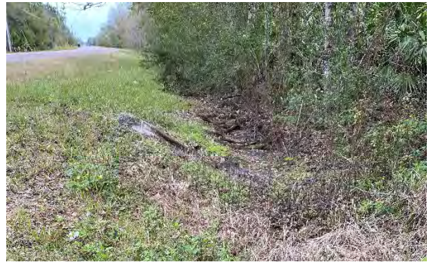
Upstream of 18" RCP crossing Starry Street at approximately Station 1464+50 BL SR 528 east of the Dallas Boulevard and Starry Street Intersection. MES cracked. (facing east)
