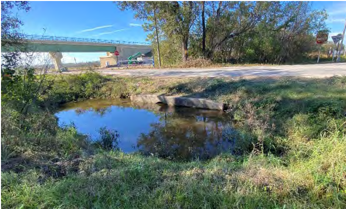
Upstream of double 29" x 45" ERCP on the east side of Dallas Blvd just across from the existing off-ramp (facing southwest)
