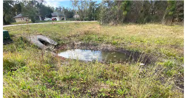
Downstream of 18" RCP crossing Starry Street at approximately Station 1464+50 BL SR 528 east of the Dallas Boulevard and Starry Street Intersection. MES cracked. (facing southwest)
