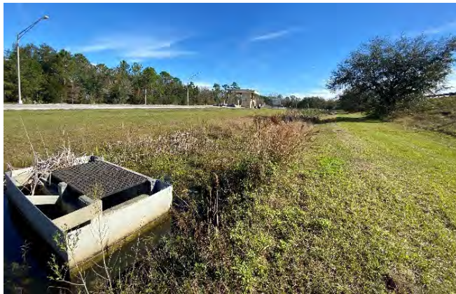
Pond 403-1A and control structure within the infield of the existing on-ramp and SR 528 westbound. Vegetation in skimmer. (facing east)
