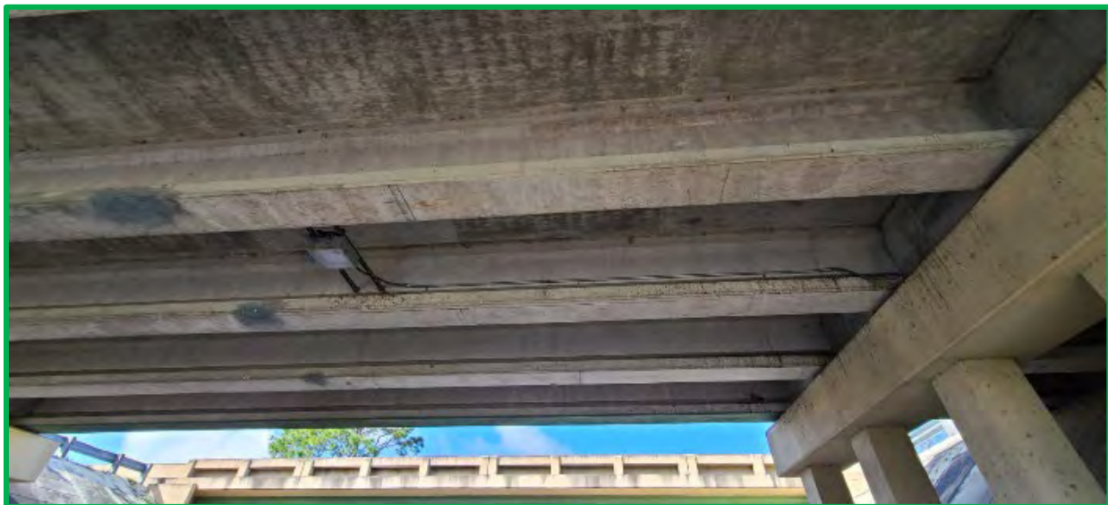
Figure 11 - Bridge-Mounted Underdeck Fixtures
