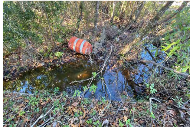
Downstream of double 29" x 45" ERCP on the west side of Dallas Blvd just south of the off-ramp (facing west)
