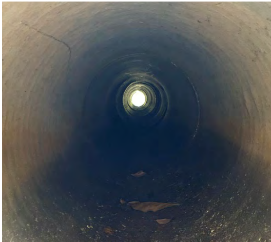
Inside pipe on upstream side of 18" RCP crossing Starry Street. Okay condition. (facing north)
