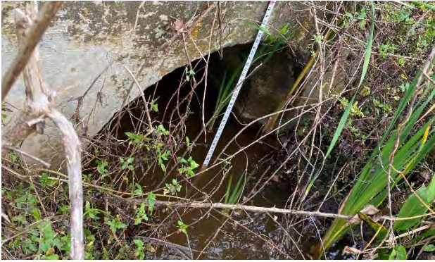
Downstream of 36" RCP Cross Drain at Station 1444+00 BL SR 528. 14" of water observed. (facing northeast)
