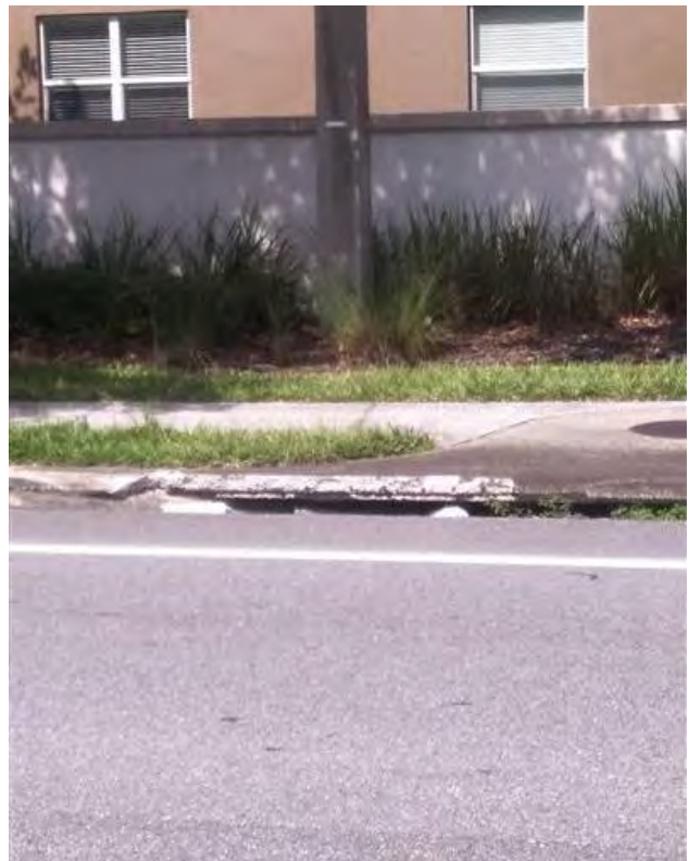
Figure 19: Damaged Inlet – SR 551 Goldenrod Road.
