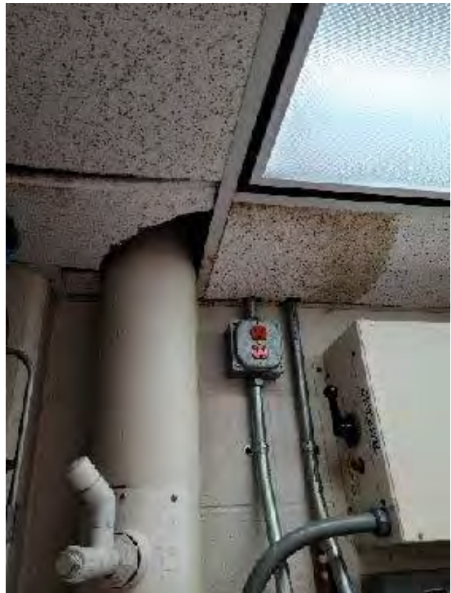
Figure 12: Damaged ceiling tile - Landstar off ramp
