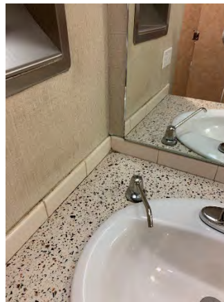
Figure 48 Building Headquarters Third Floor (Women's RR)
