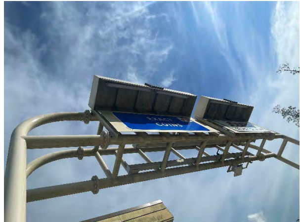
Figure 64 ICP Ramp Off
