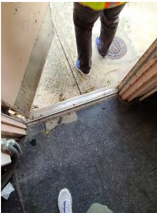
Figure 35 Conway Ramp Off
