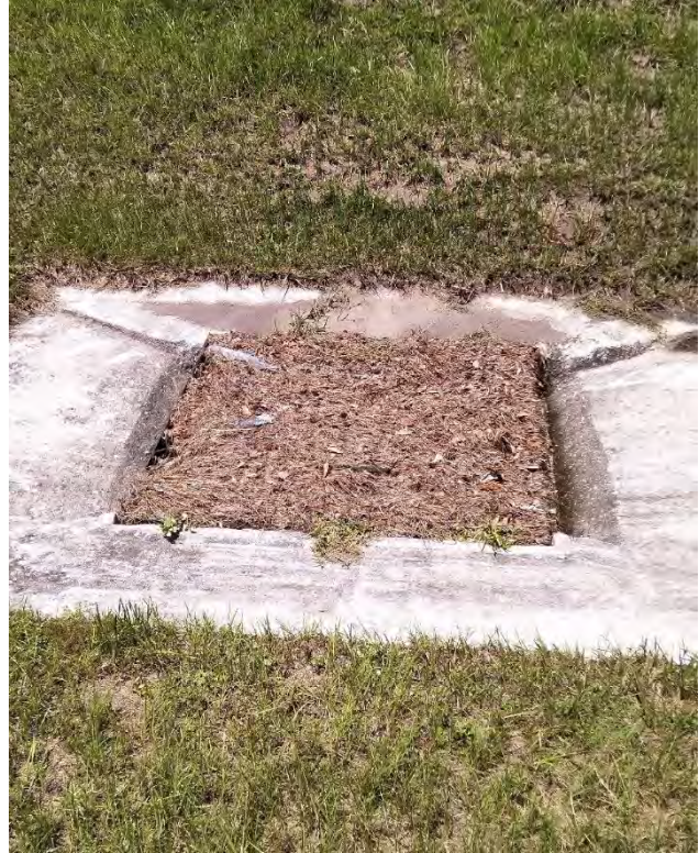
Figure 13: Debris covering drainage structure grate - south of Yothers Road.
