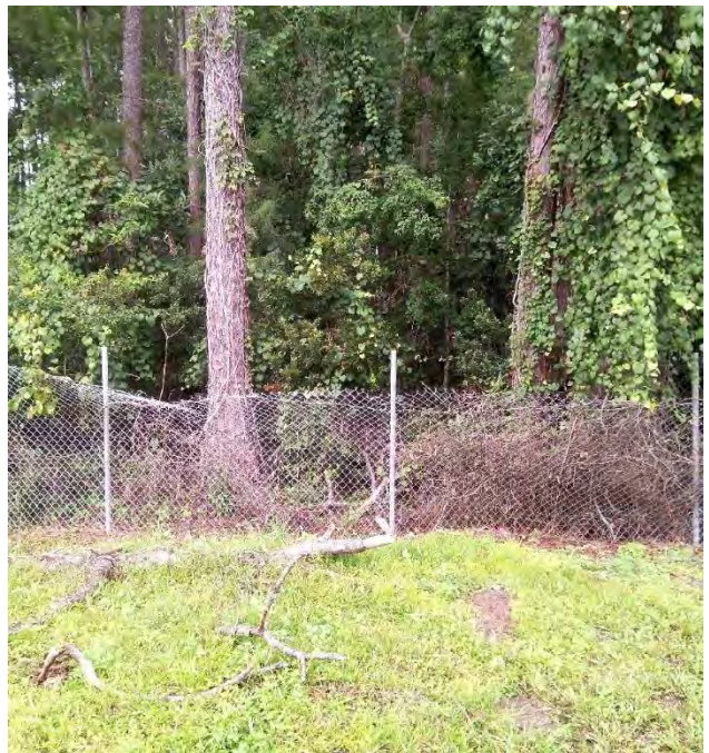
Figure 4: Damaged right-of-way fence - SR 408 and Dean Road
