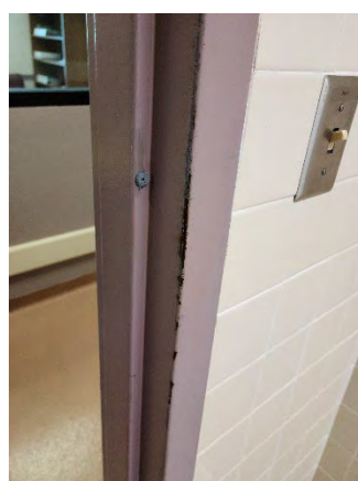
Figure 6 Coral Hills Mainline
