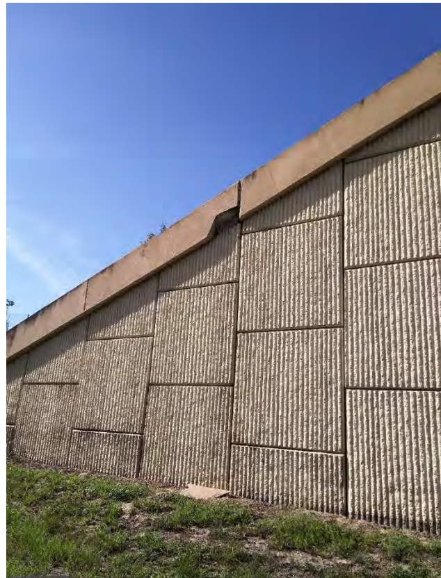
Figure 16: Damaged MSE wall coping - Ocoee Apopka Road
