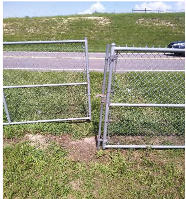
Figure 14: Damaged fence gate Plymouth Sorrento Road- Plymouth Sorrento Road.
