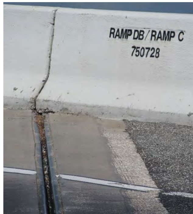
Figure 8: Debris at bridge abutment and shoulder - SR 414.
