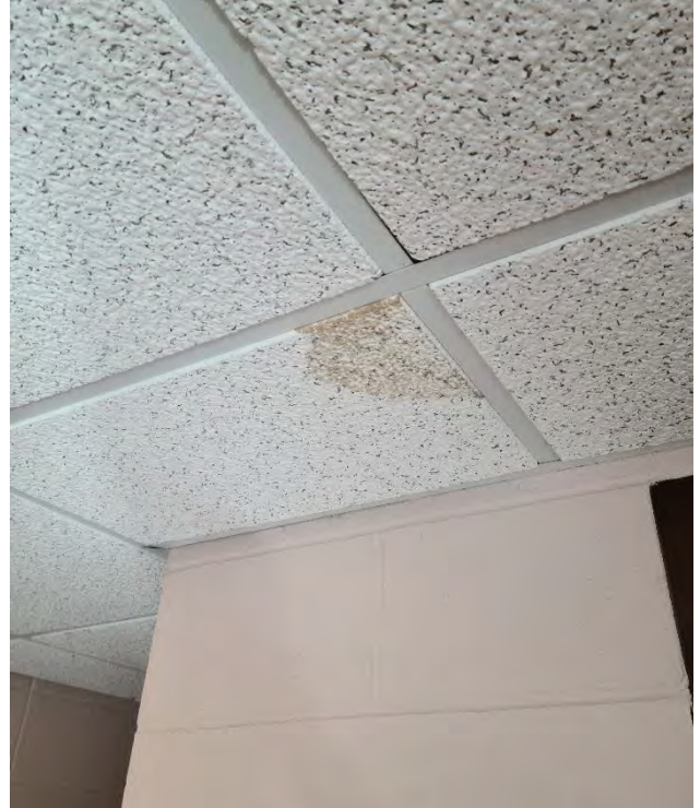
Figure 9: Damaged ceiling tile - SR 414 Keene Road off ramp.
