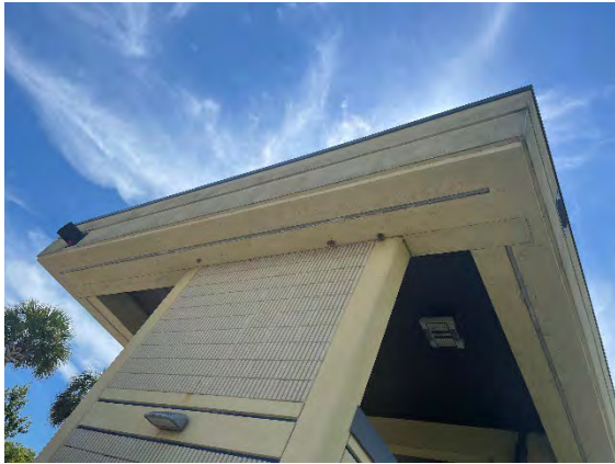
Figure 43 Conway Ramp Off
