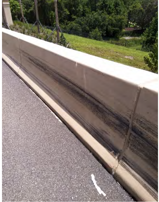
Figure 5: Scuffed barrier wall - SR 408 and Alafaya Trail
