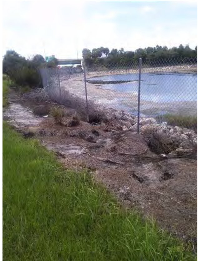
Figure 18: Minor erosion – Goldenrod Road Interchange.
