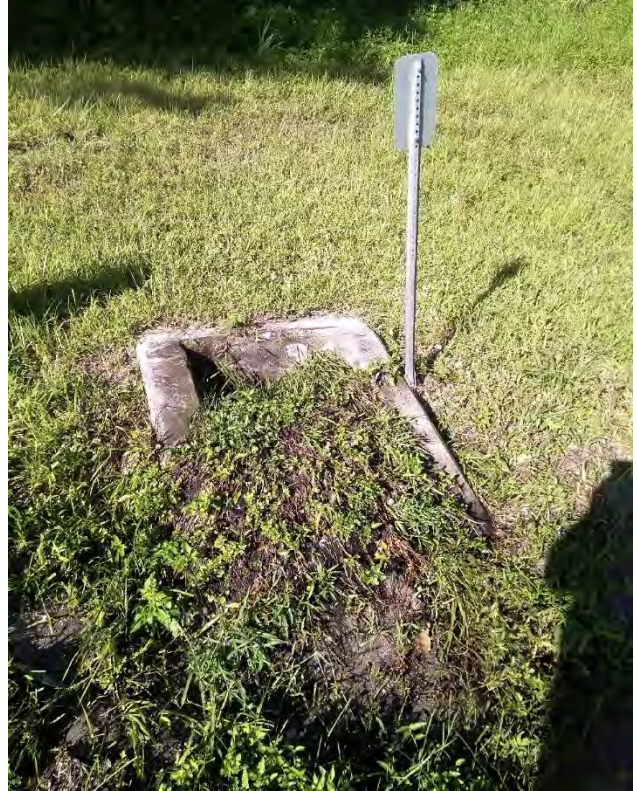
Figure 3: Mitered end structure needs vegetation and sediment cleared.
