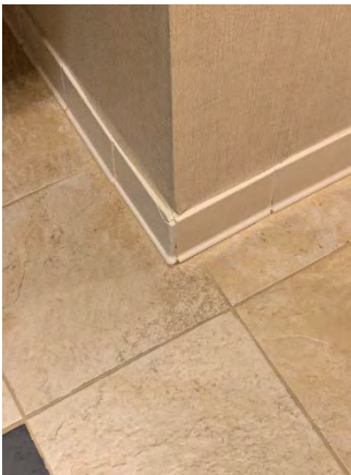
Figure 47 Building Headquarters Third Floor (Women's RR)
