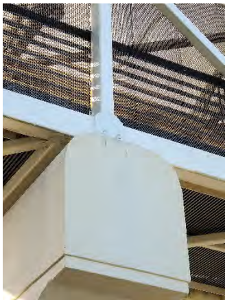
Figure 11 Coral Hills Mainline
