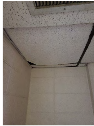
Figure 46 Hiawassee Ramp Off
