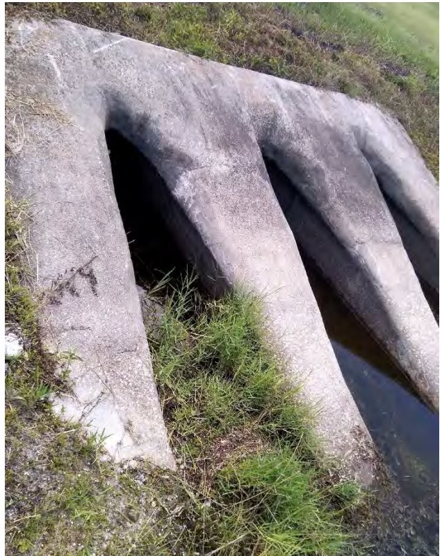
Figure 6: Sediment filled drainage structure - SR 414 pond
