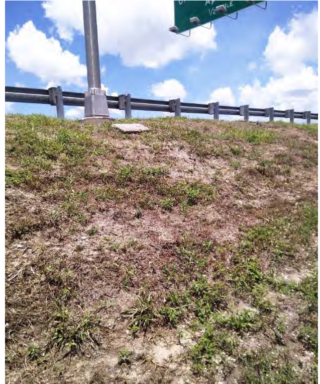
Figure 17: Minor slope erosion – SR 451.
