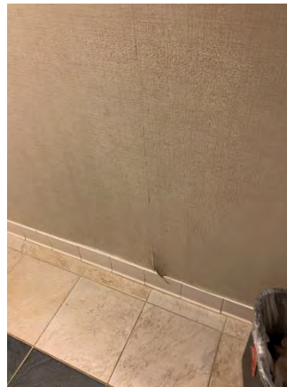
Figure 46 Building Headquarters Third Floor (Women's RR)
