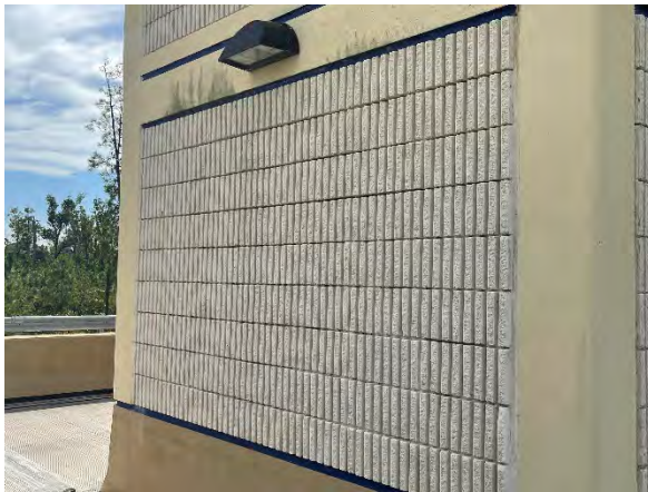
Figure 63 ICP Ramp Off
