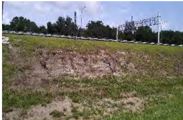
Figure 14: Front slope erosion SR 429 and Kelly Park Road.
