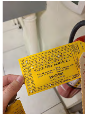
Figure 48 Conway Ramp Off
