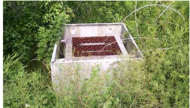
Figure 3: Damaged pond structure SR 408 and Rouse Road
