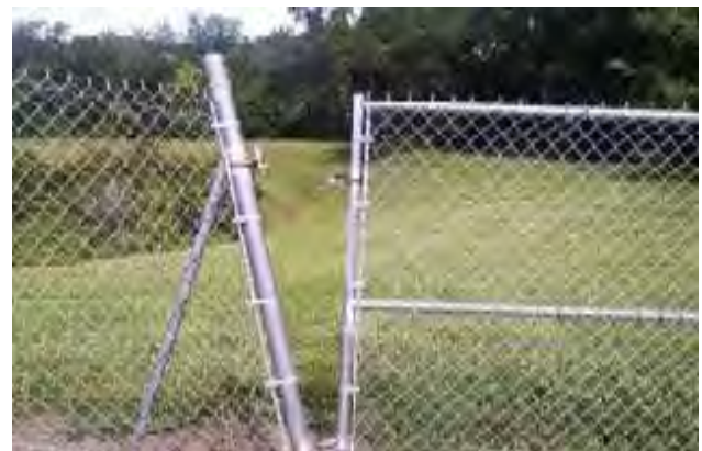
Figure 7: Leaning fence gate Hiawassee Road pond.
