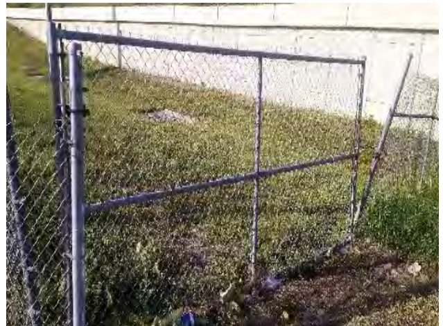
Figure 11: Fence gate damaged at Valencia College Lane.
