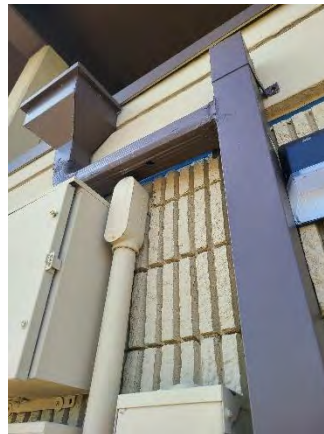
Figure 52 Conway Ramp Off
