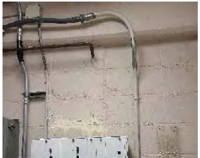
Figure 12: Curry Ford on ramp interior coatings in poor condition.
