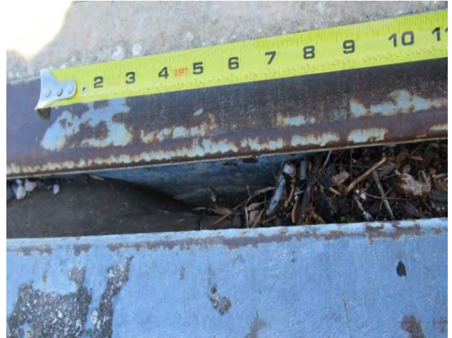
Figure 10: Joint sealant at abutment missing SR 417 over Rhode Island Woods Boulevard.
