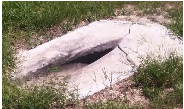
Figure 17: Damaged drainage structure SR 451.
