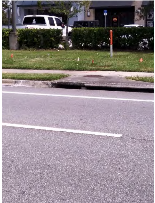
Figure 19: Damaged Inlet – SR 551 Goldenrod Road.
