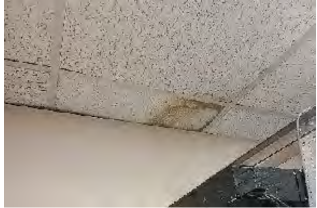
Figure 16: Water stained ceiling tile Data Room Forest Lake Mainline Plaza
