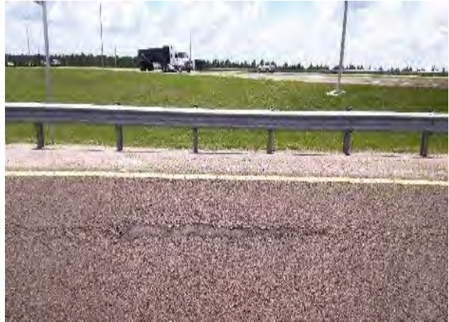
Figure 13: Pavement raveling Schofield Road ramp.
