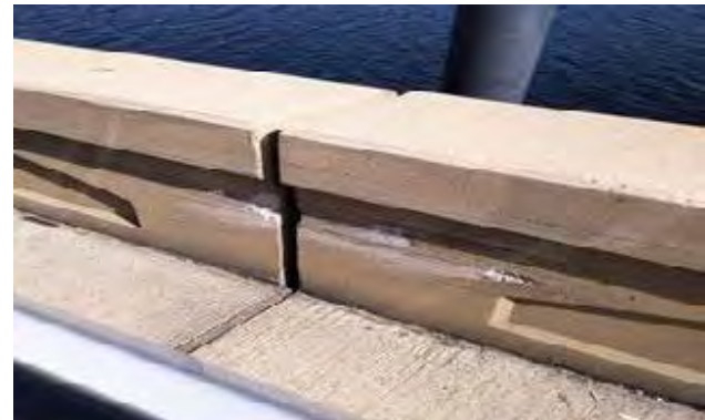
Figure 4: Damaged bridge traffic railing coating over Lake Underhill
