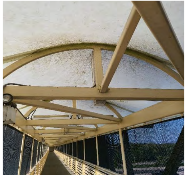
Figure 8: Mold present on canopy Coral Hills Mainline Plaza pedestrian bridge.
