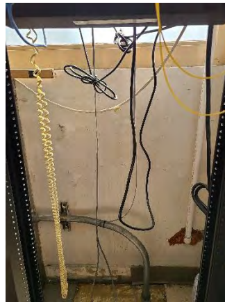
Figure 34 Dean Ramp On
