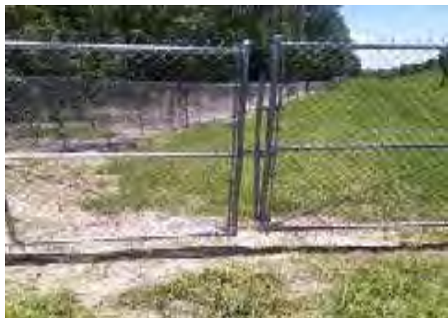
Figure 15: Gate missing lock and chain SR 429 south of Mt. Plymouth Road.
