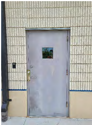
Figure 45 Conway Ramp Off
