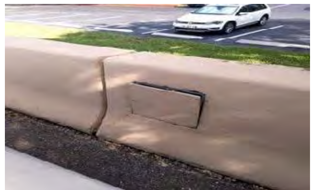
Figure 5: Damaged junction box cover Rosalind off ramp
