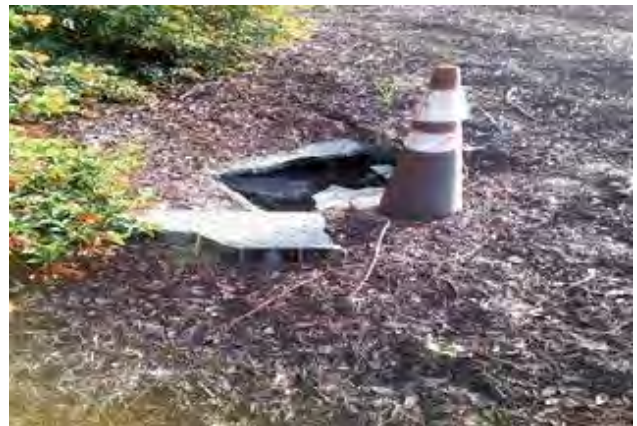
Figure 6: Damaged splice box Keene Road exit Ramp
