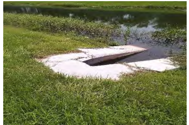
Figure 9: Overgrown drainage structure SR 417 north of Berry Dease Road
